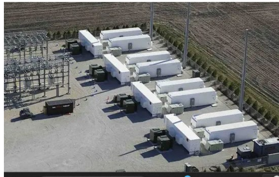
Figure 24: Typical container BESS (external) 9 :
