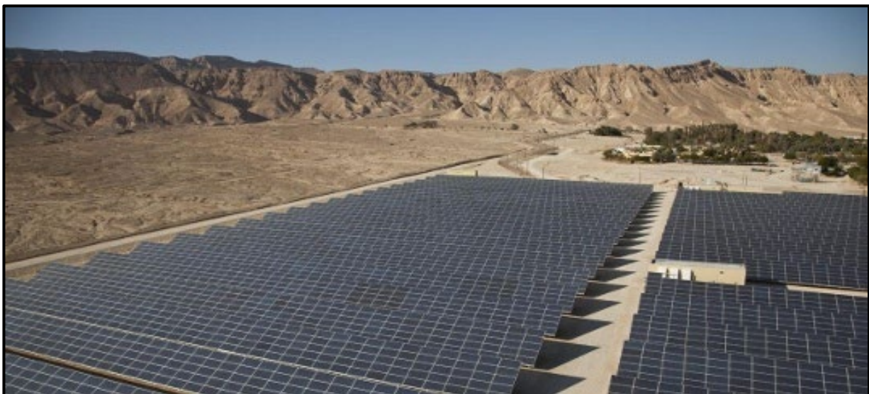
Figure 3: Typical Power Arrays Composed of PV Panels
