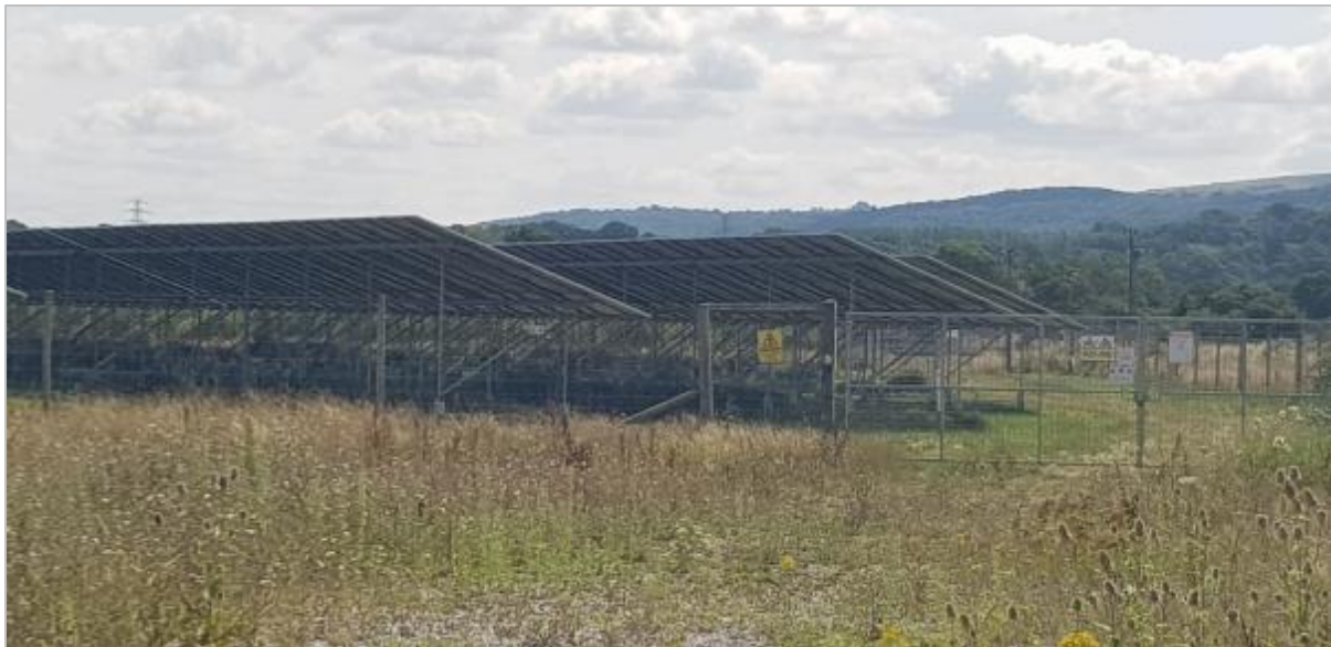
Figure 2-12. Typical Fence and CCTV System at a UK PV Facility
