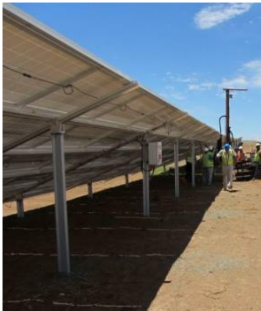
Figure 2-6. Example of fixed tilt solar panels on H-style steel piles
