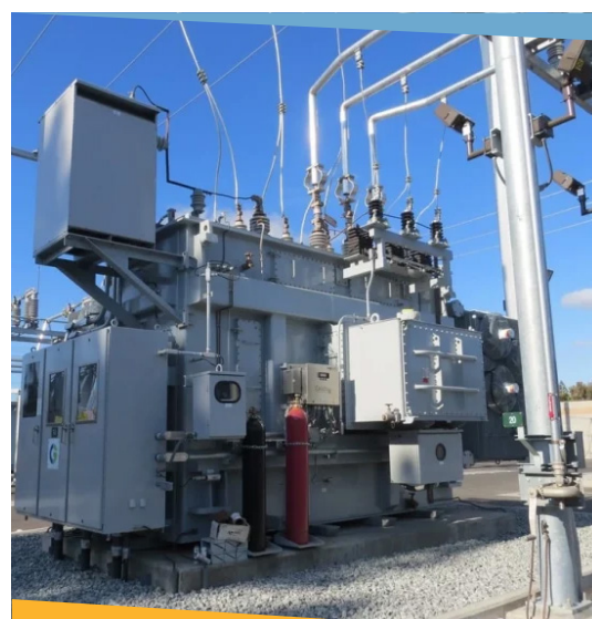
Example of Transformer
