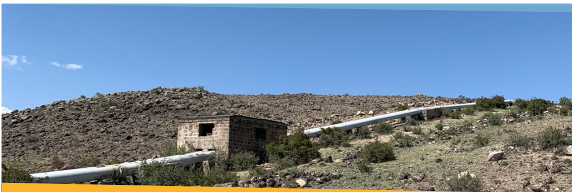
Water Pipeline and Pump Building at the Project Site
